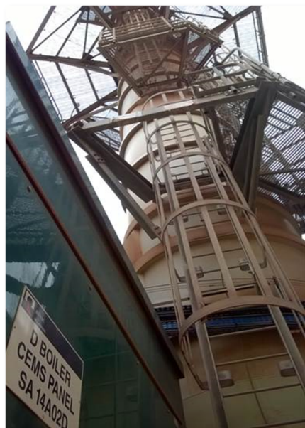
Figure 2. Location of CEMS adjacent to gas boiler stack.
