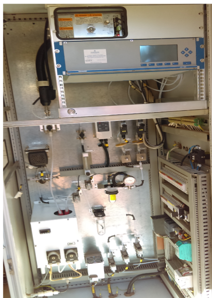
Figure 3. Emerson CEMS for gas boiler stack emissions monitoring.
